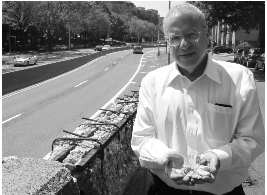
Assemblyman Dinowitz has asked the New York State DOT to repair severely deteriorated retaining walls along Henry Hudson Parkway between West 231st and West 235th Streets. He is shown here holding part of the wall. Read more on Page 2!
