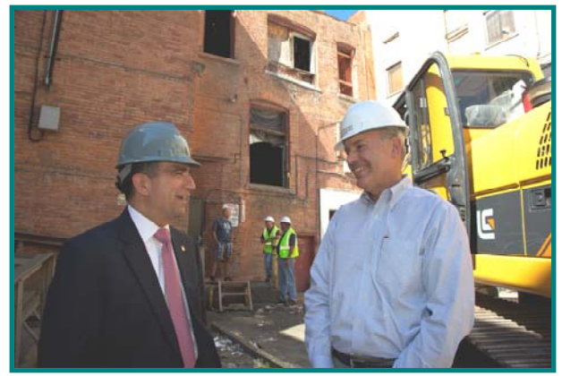
Assemblyman Magnarelli speaks with David Nutting, President, VIP Structures, after part of the Bond Building was demolished.
